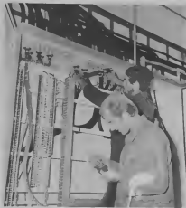
TECHNICIANS WORK ON tie-in of LCAH controlhouse with centralized refining controlhouse. TECNICIONAN TA conecta LCAH Controlhouse cu controlhouse central di refinacion.
